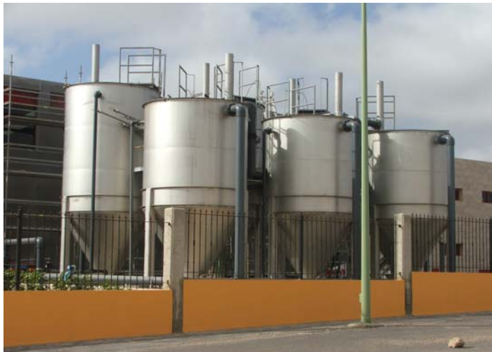
Tertiary filters at Puerto del Rosario
